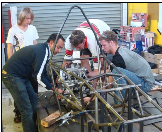
Mr Hiten Parmar (Front left) with the NMMU racing team at the VW racing premises during construction of the vehicle frame
